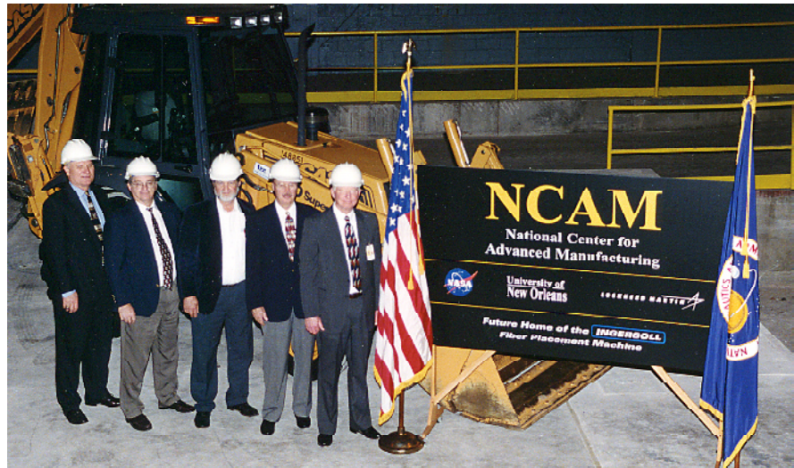
Rey Abadie (left), Dennis Deel, Randy Tassin, UNO Engineering Dean John Crisp and NASA Manager John White check the groundbreaking for the fiber placement machine.
