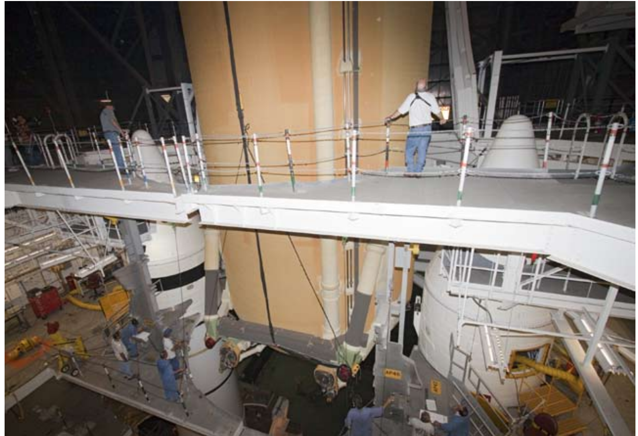
Workers at KSC go through the delicate process of aligning shuttle elements during the mating of ET-137 with the Solid Rocket Boosters.
