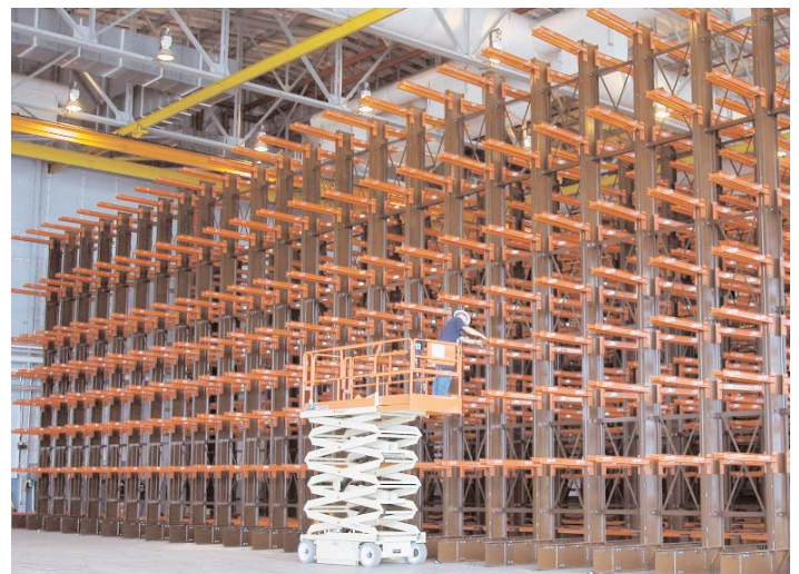
A subcontractor employee inspects a support member in the cavernous storage system currently under construction in Building 303 that will house thousands of Space Shuttle Orbiter inventory items at Michoud.
