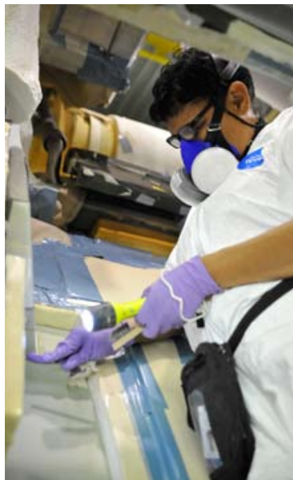
TPS mechanic Theresa Rivera works final closeout on the +Y vertical strut, which is part of the aft interface hardware.
