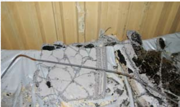
Katrina's debris lodged against ET-122 in Cell A.
