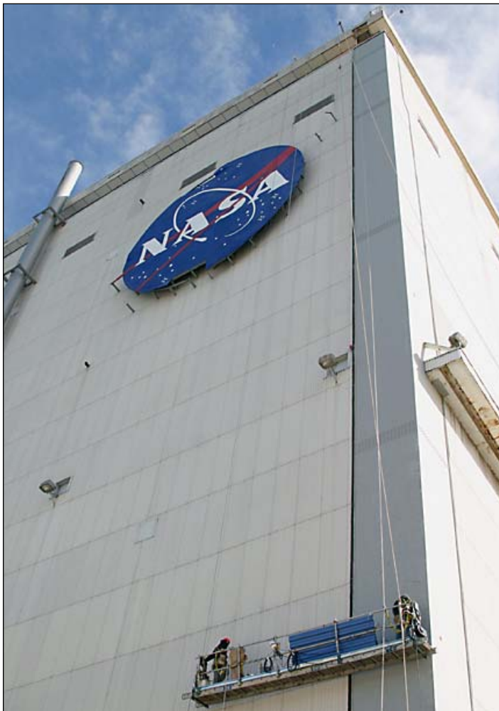
Contractors replace blown-out VAB skylights Ironworkers from AC Dellovade Company make their way up the side of the Vertical Assembly Building to replace the remaining skylights with blue panels that will surround the top of the VAB.
