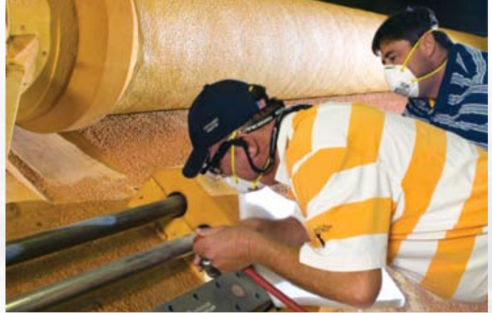
Wendell Cannon, Thermal Protection Systems mechanic, routs out damaged foam from an Ice Frost Ramp on ET-122’s Liquid Hydrogen Tank in preparation for a PDL pour repair as Quality Control inspector Michael Gough looks on.
